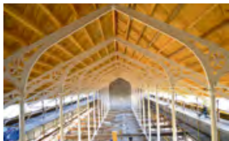
A 200-year-old former Dundee jute mill that was saved from collapse
